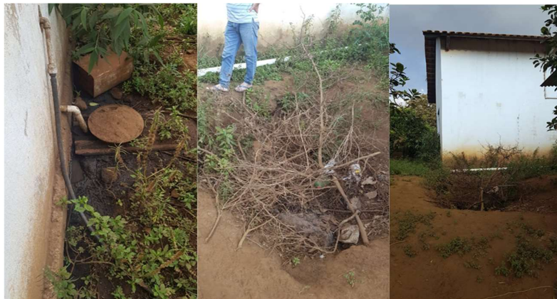
Figure 3: Grease trap and trench for disposing of the school's wastewater.
