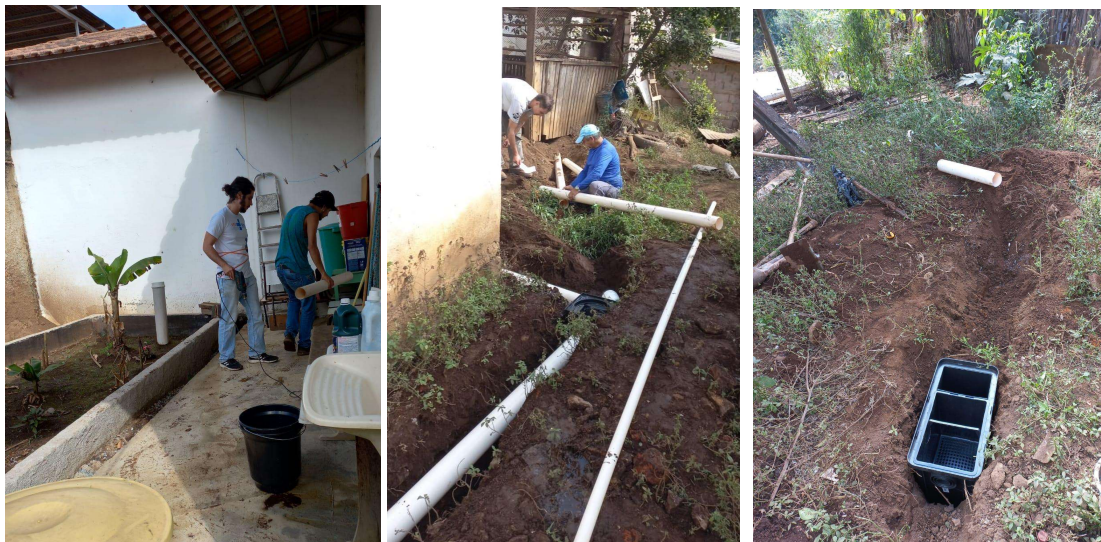
Figura 7: records of the step to connecting the bathroom pipes with the TEvap and installing the grease trap (GT) and infiltration trench (IT).
