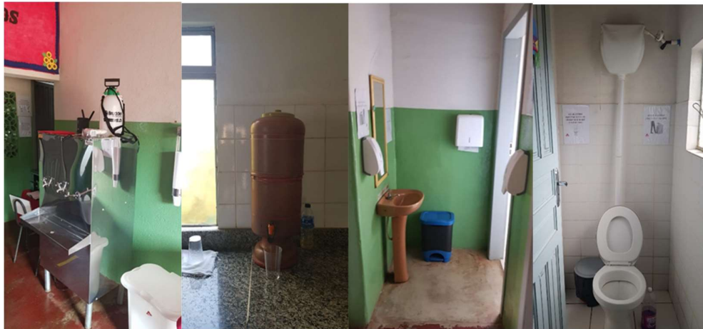
Figure 2: Water tap, filter, washbasin, and toilet..
